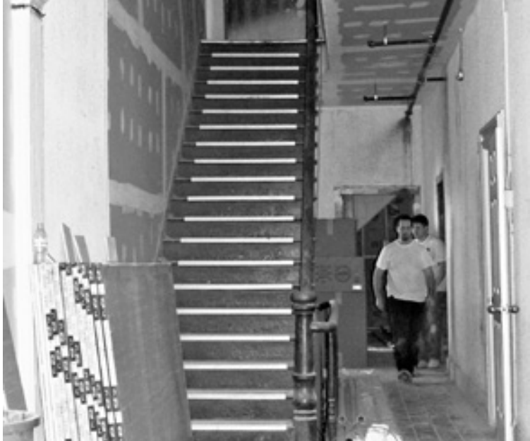
David George, Jr., son of the hotel owner, and Blane Bidle, Midview Properties, help with the ongoing renovation of the Emmitsburg Hotel.
